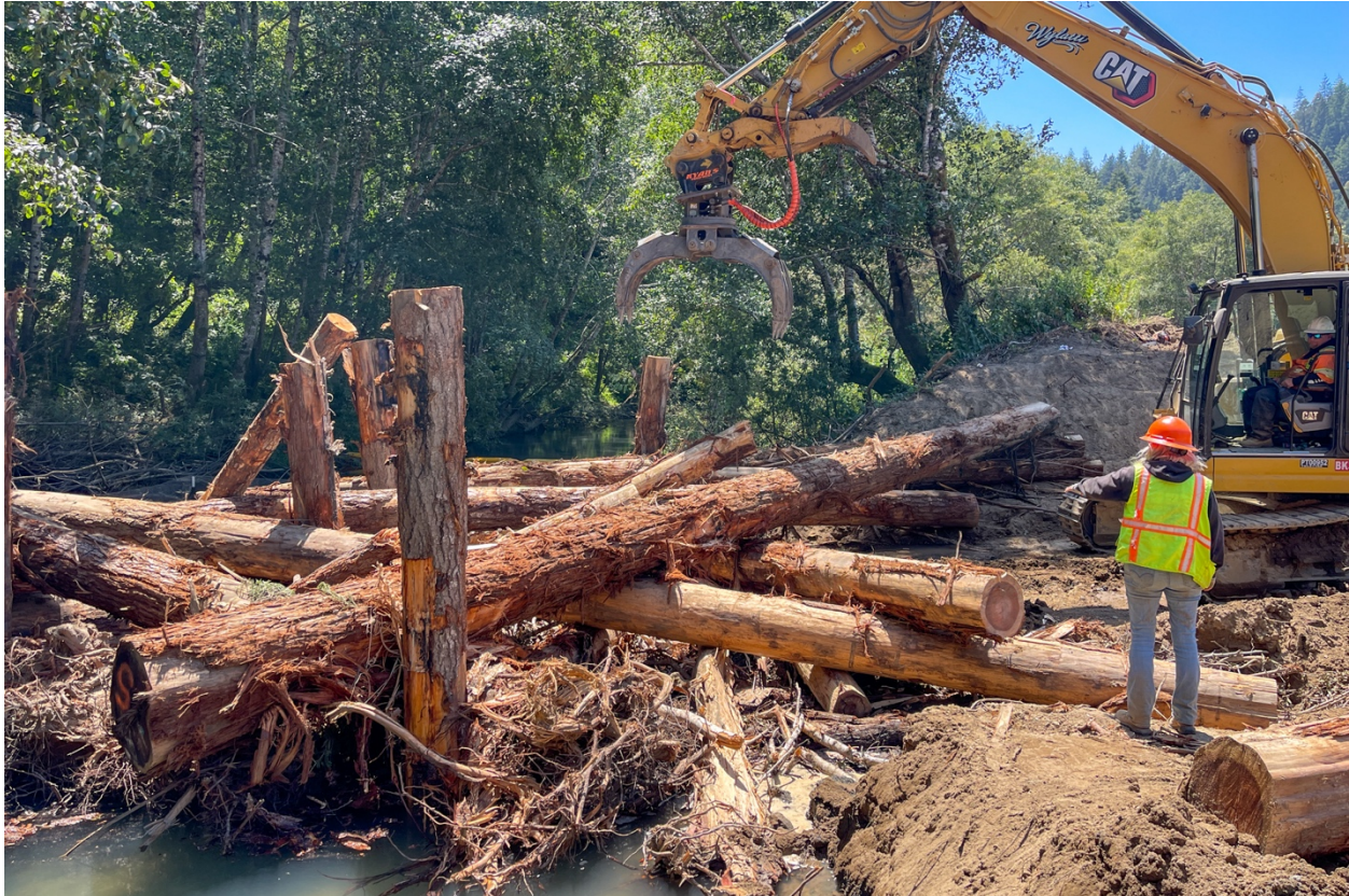
Building an engineered log jam on the Ten Mile River. Credit: The Nature Conservancy
